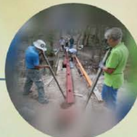
Lindheimer Chapter members repair a trail bridge over a slough that feeds into the Guadalupe River.
