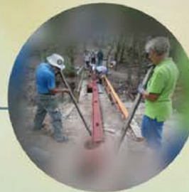
Lindheimer Chapter member repairs a trail bridge over a slough that feeds into the Guadalupe River.
